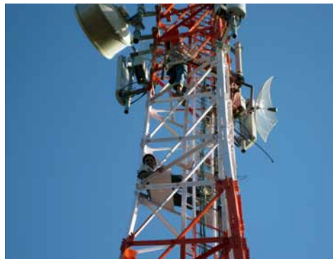
Network team setting up antenna on NCell tower in Rupesh Kanda, Doti
